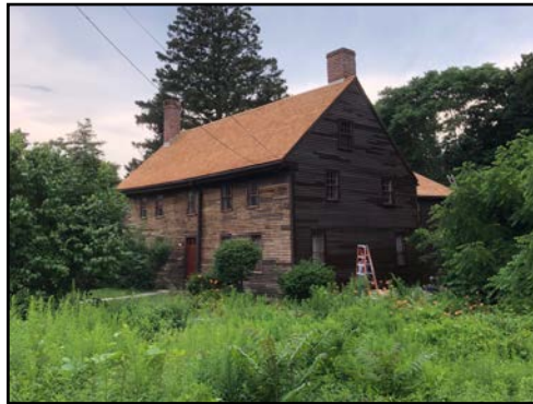
Historic New England recently completed a project update the 1678 Tristram Coffin House on High Road, Newbury, with a matching grant through the Mass. Historical Commission. Here, retaining of the clapboards is almost done.
